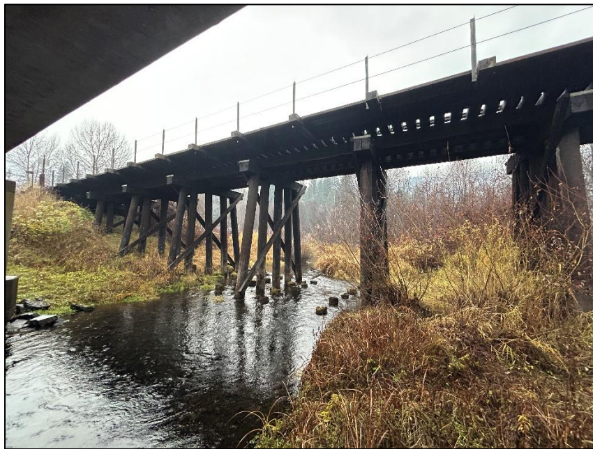
Photo C2: Highway 3B Outdated Bridge
