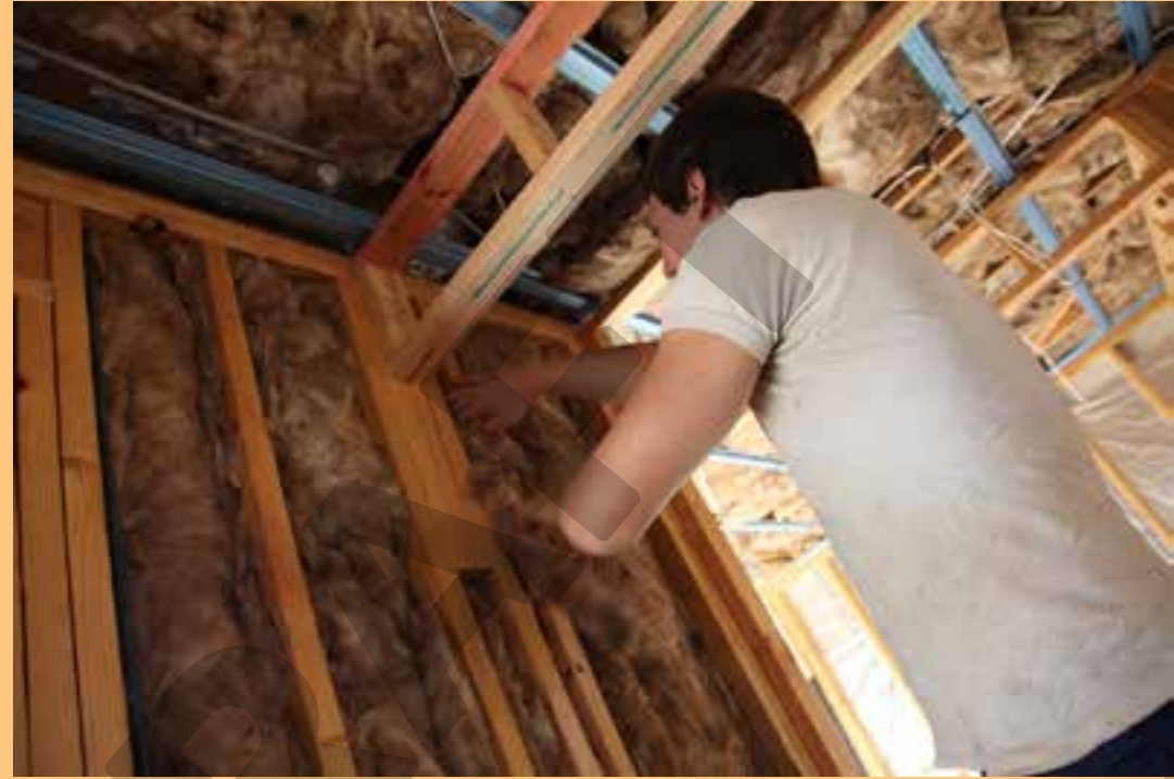
Adding insulation in crawlspaces, basements, and attics is one of the easiest ways to increase the efficiency and comfort of your home.
